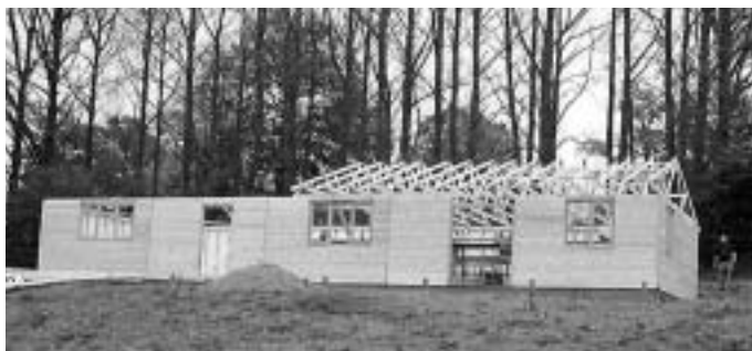
The almost complete clubhouse for Ebrington Cricket Club, near Chipping Campden. (See page 21).
